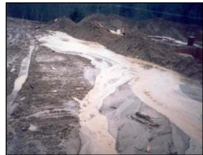
Sediment loaded stormwater runoff
