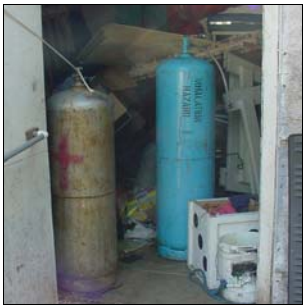
Ammonia tanks used in manufacturing
